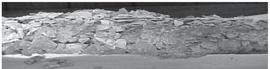
Portion of a scale-encrusted boiler tube from No. 27
