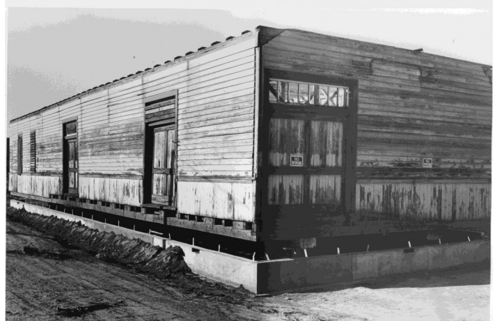
August 1, 1983. Wabuska Depot being set on its new foundation. Daun Bohall photo, NSRM
